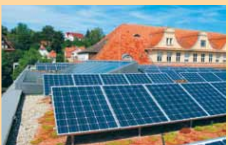
Roof with fully-installed solar energy system.
