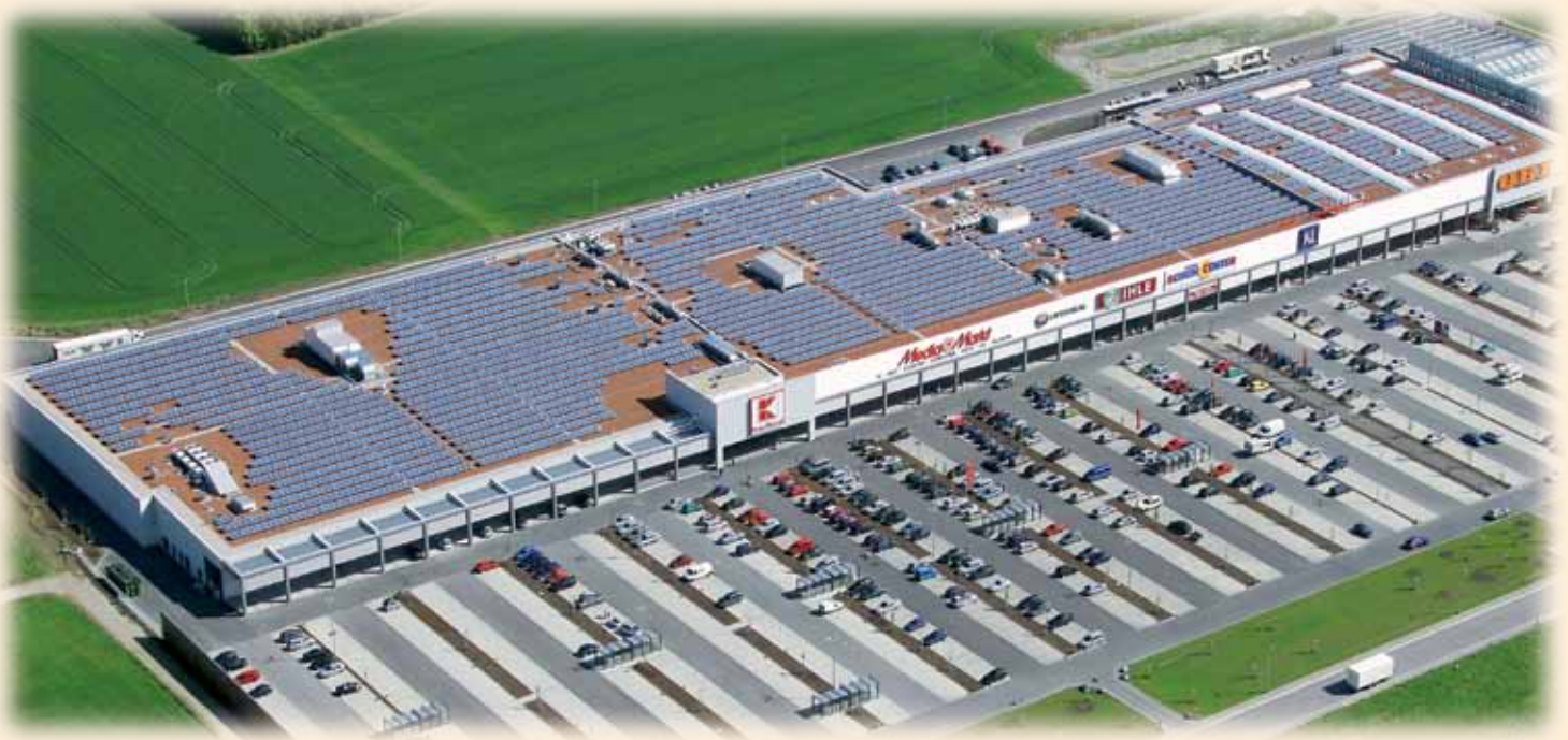
Photovoltaic plant on the roof of the "InCenter" shopping mall in Landsberg/Lech, Germany.
