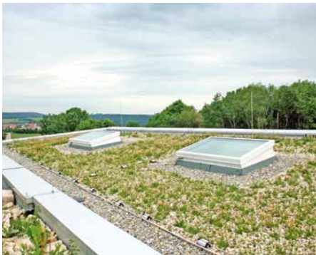
The substrate used is a special mixture of lime grit, lava and top soil.
