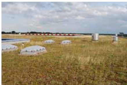
A conventional extensive green roof build-up (“Sedum Carpet”) evaporates 20–50 l/d in the summer heat.
