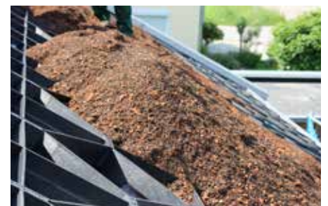
The system substrate “Heather with Lavender-light” is, e.g. delivered in a silo tanker. It is then blown onto the roof until the Georaster® elements are filled and covered up to about 10 mm over their upper edge.
