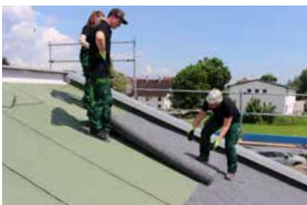
The roof area to be greened is sealed with rolls of waterproofing membrane that have been tested for their root-resistance in line with FLL procedures.
