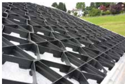
Once the area has been covered with the Protection Mat WSM 150, the Georaster® elements are installed, starting from the bottom up.
