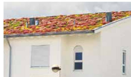
A shear barrier is placed just above the eaves on this monopitch roof, which is drained by means of an outer-lying gutter.
