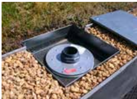
The limiter element is protected beneath the inspection chamber and regulates the slow discharge of water. At the same time, it acts as an overflow.
