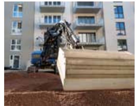
Thanks to the stable ZinCo system build-up with RSX 80, using diggers to apply the substrate is not a problem. © Strassen- und Tiefbau Urban GmbH
